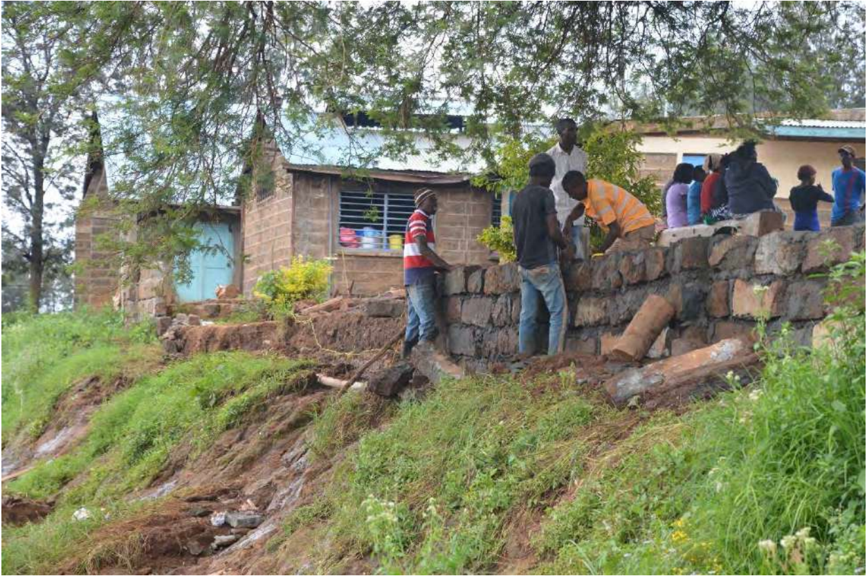
Solai Victims re-building one of the school walls which was destroyed by spillage from the Solai Dam
