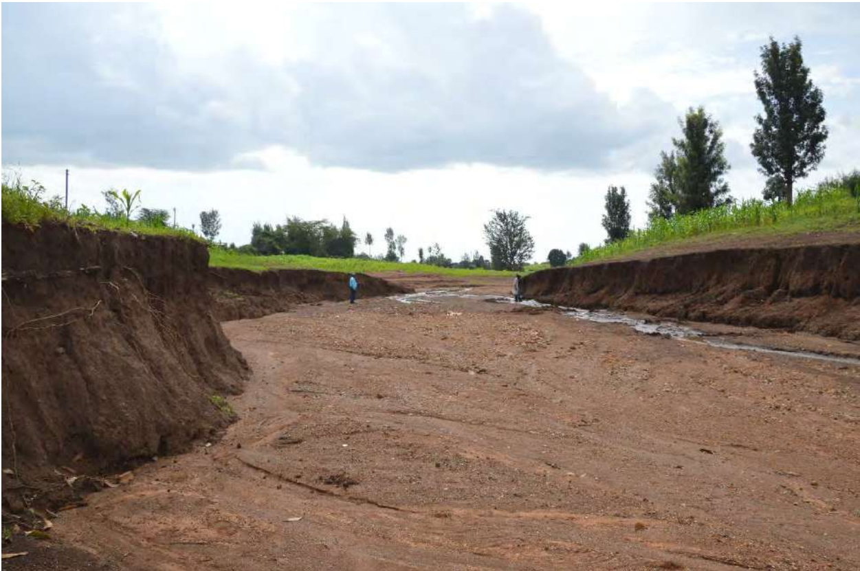
Deep gully erosion caused by water from the Solai Killer Dam.
