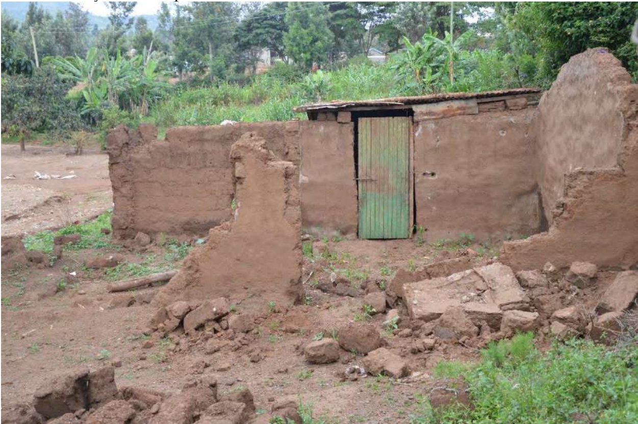
A semi-permanent building in Nyakinyua village, Solai destroyed by waters from the killer dam.
