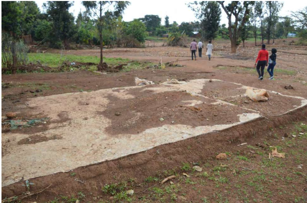
The foundation of one of the buildings which was swept away by water from the dam.
