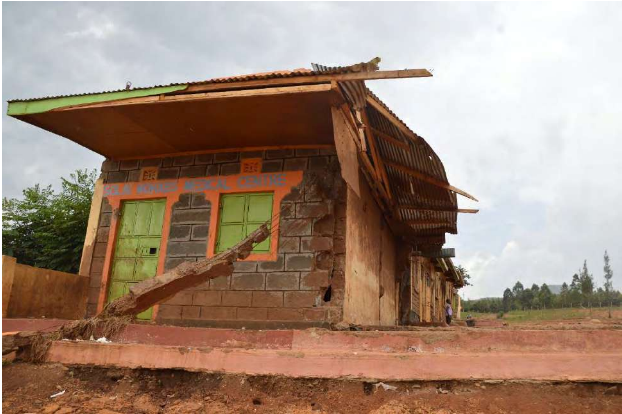
Private medical center damaged by the Solai dam waters.
